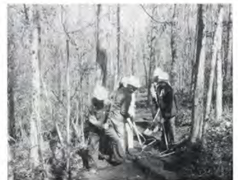
Local unemployed people were hired to build the Crooked Creek Nature Trail. They did much of the work by hand.
